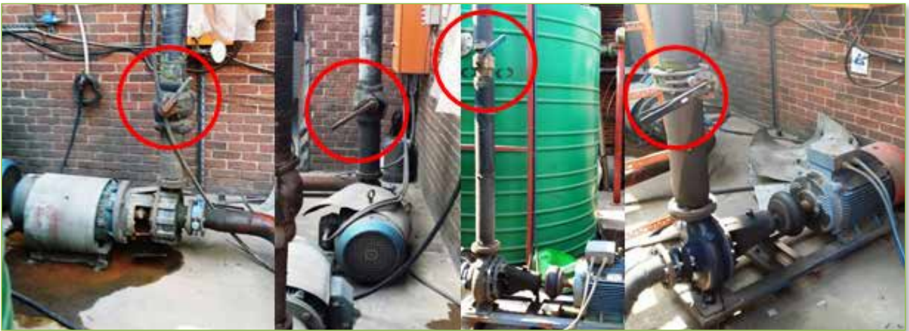
Figure 17. Pictures of throttled pump systems
