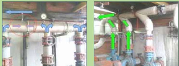
Figure 1: Cooling Water Pumps Configuration
