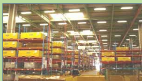
Figure 3: Daylight harvesting in Imported Parts Warehouse
